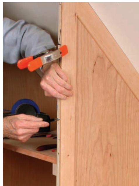
Fit the front edge too. Once the wall side of the frame is profiled, set it in place and use the plywood divider to run a line along the back side of the end cap. Cutting to this line will make sure the front is perfectly flush with the edge of the plywood, which is crucial because the face frame has to land there.
