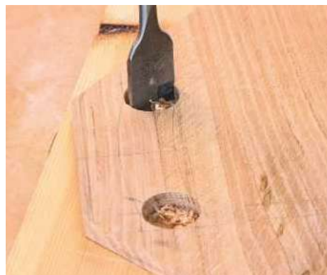
24 Mark hole centres and cramp the board to some backing material. Bore ends of the cutout with a 25mm flat bit
